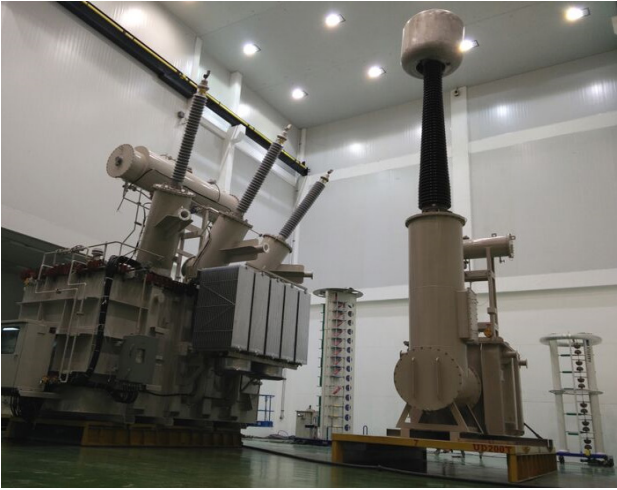
230kV Power Transformer (Left) 400kV Testing Transformer (Right)
