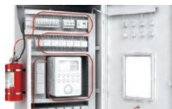
Electrical Cabinets Suppression
